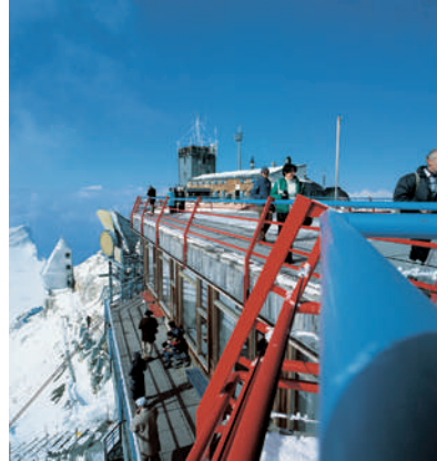
Siemens Energy transformer on top of the Alps Mountain.
